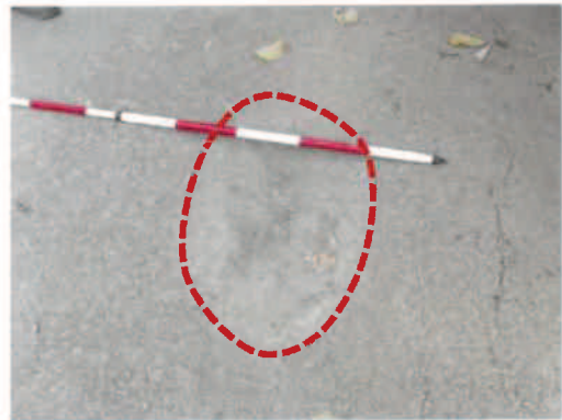
⑫路面の陥没
